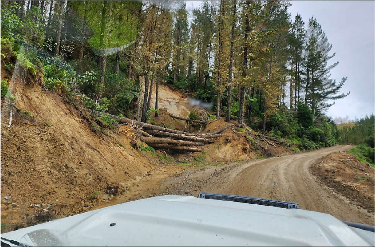
Photo 2: Damage after Cyclone Hale in Portview Group Forest, Gisborne (photo May 2023).
