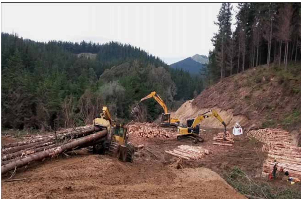
Skidder pulling cut trees to the landing for processing into logs, which are then stacked ready for loading onto trucks. Photo April 2016
